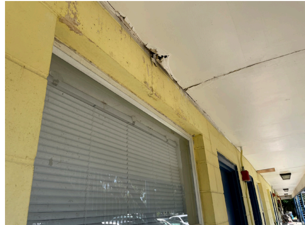
Figure 14 - Damaged soffit NE Building
