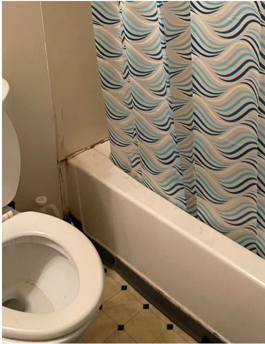
Figure 36 - Typical tub condition
