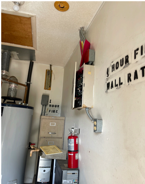
Figure 34 - Utility room SW building
