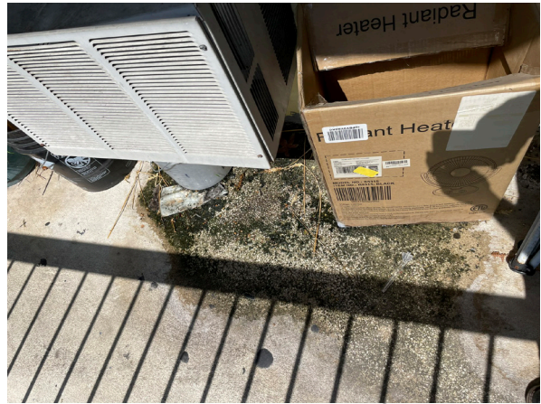
Figure 19 - AC unit condensation overflow SW building
