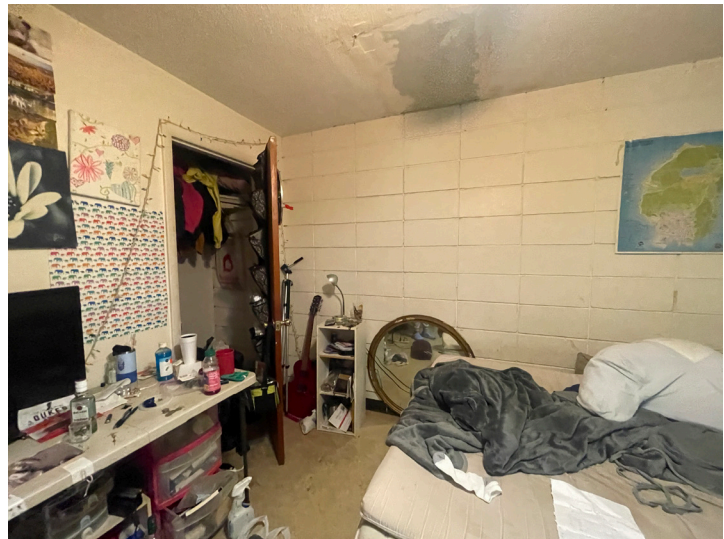
Figure 33 - Repaired water leak above second bedroom in larger unit SW building
