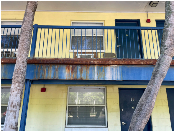
Figure 4 - Rusting Steel Structure NE Building
