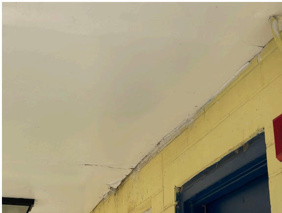
Figure 18 - Paint peeling on lintels above windows
