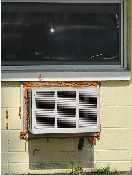
Figure 17 - Typical AC unit SW building
