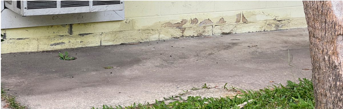
Figure 10 - Flood Damage in NE Building
