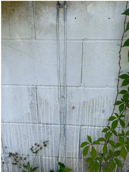
Figure 11 - Stair stepping in CMU walls
