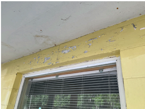
Figure 15 - Paint peeling on lintels above windows
