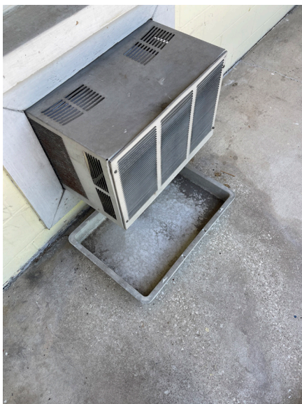
Figure 9 - Typical AC Unit
