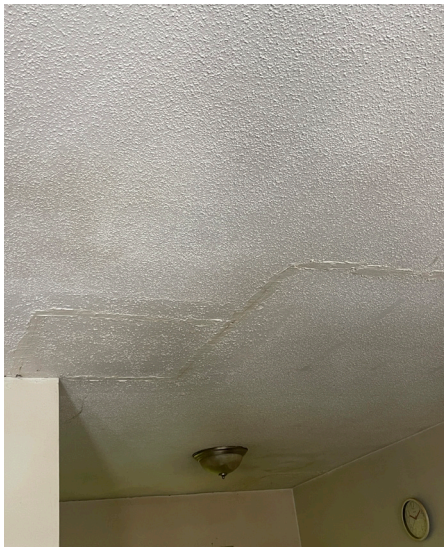
Figure 32 - Repaired water leak above dining room in larger unit SW building
