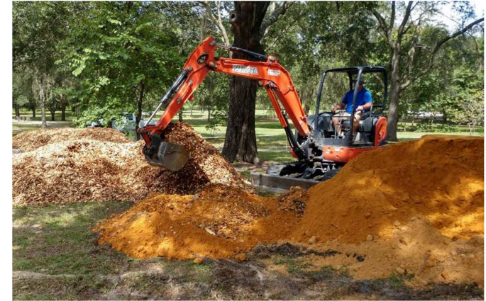
This photo shows the different materials that were put under the drainfield of the INRB system at Poe Springs County Park.
