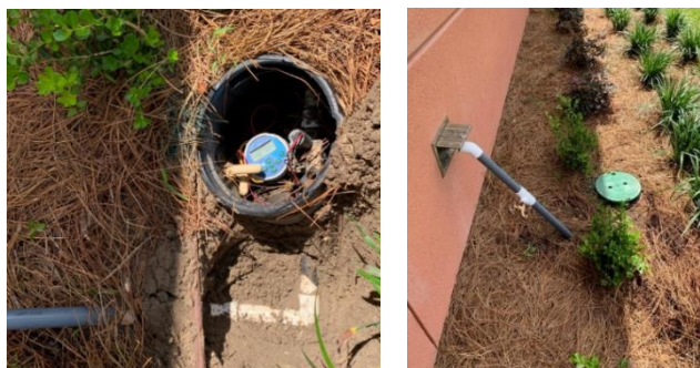
Valve timers located in valve box.
