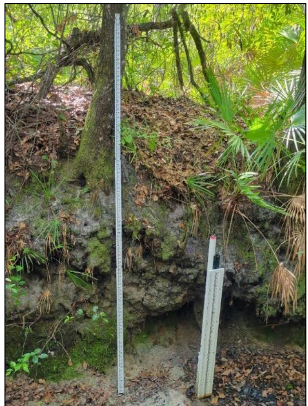
Figure 12. Incised channel near the staff gauge downstream of the southern culvert on NE 221 st Street.
