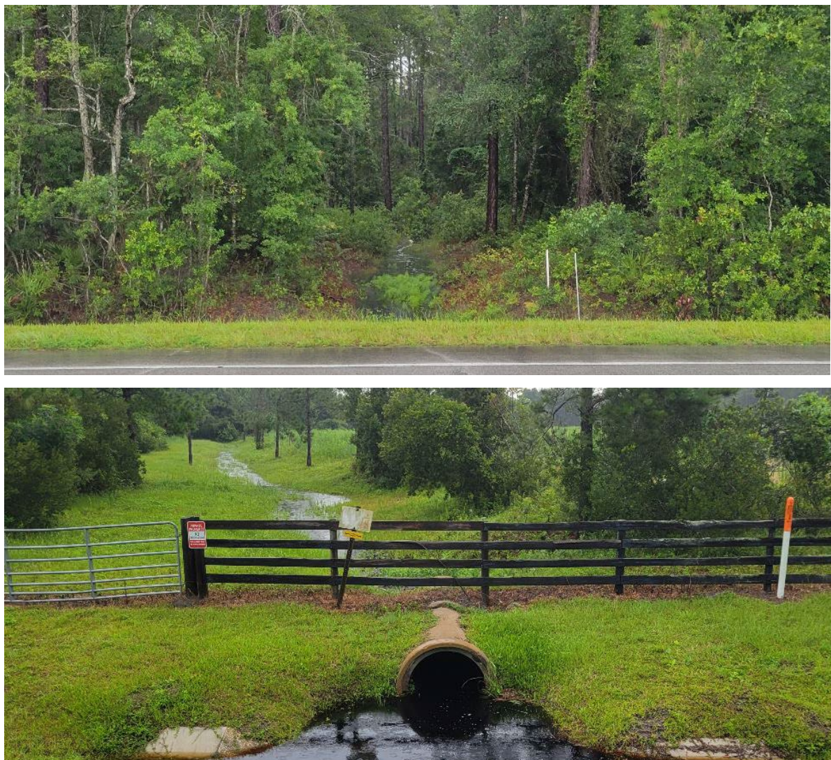
Figure 23. Water flowing from the forested parcel south of SR 26 (top picture) onto the agricultural parcel north of the highway (bottom picture). Water was also flowing from the roadside ditches on either side of SR 26.
