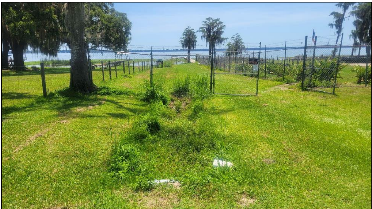
Figure 26. Outfall from the stormwater collection system along NE 100 th Avenue that discharges into a grass swale before reaching Santa Fe Lake.
